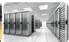
• Data Center & Server Room
